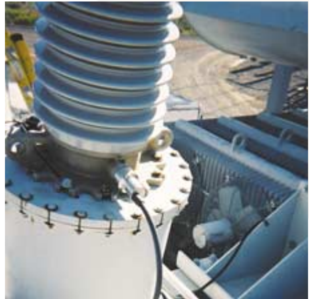
Sensor installed in capacitor tap on bushing
